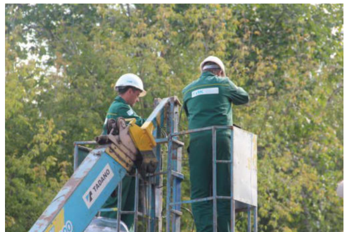
Employees of the Department of CalW carry out high-rise works at the customer's facility
