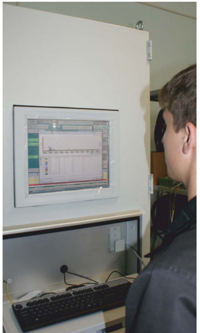
Assembly and configuration of the TIK-RVM system cabinet
